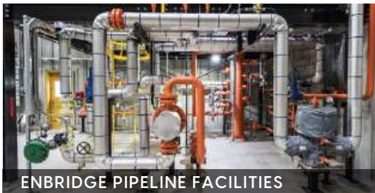
ENBRIDGE PIPELINE FACILITIES
