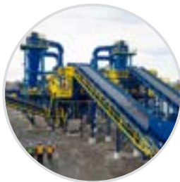
NON-FERROUS & FERROUS PROCESSING ↗
